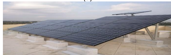
Figure 1. Installed grid-connected PV system. (a)schematic diagram, (b) capture of the PV system.
